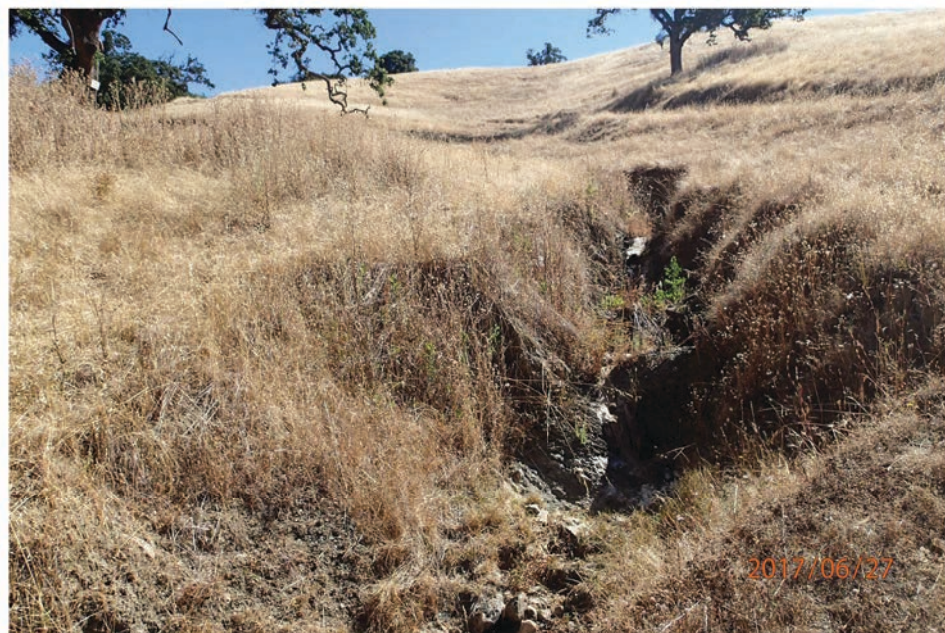
1 Headcut below Roadway at Station 1.JPG
