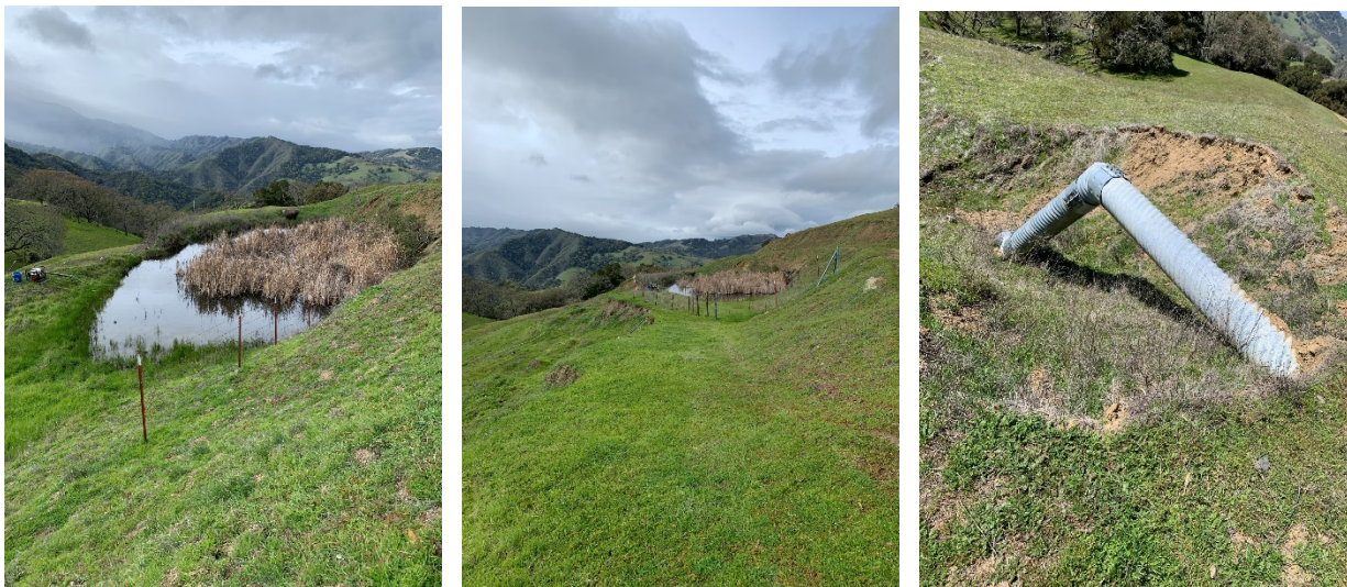
Figure 2. Pond RC-07 – (L-R) Looking down from the road (pump visible), Slumping Hillside below Embankment, Erosion and Scour around outlet pipe
