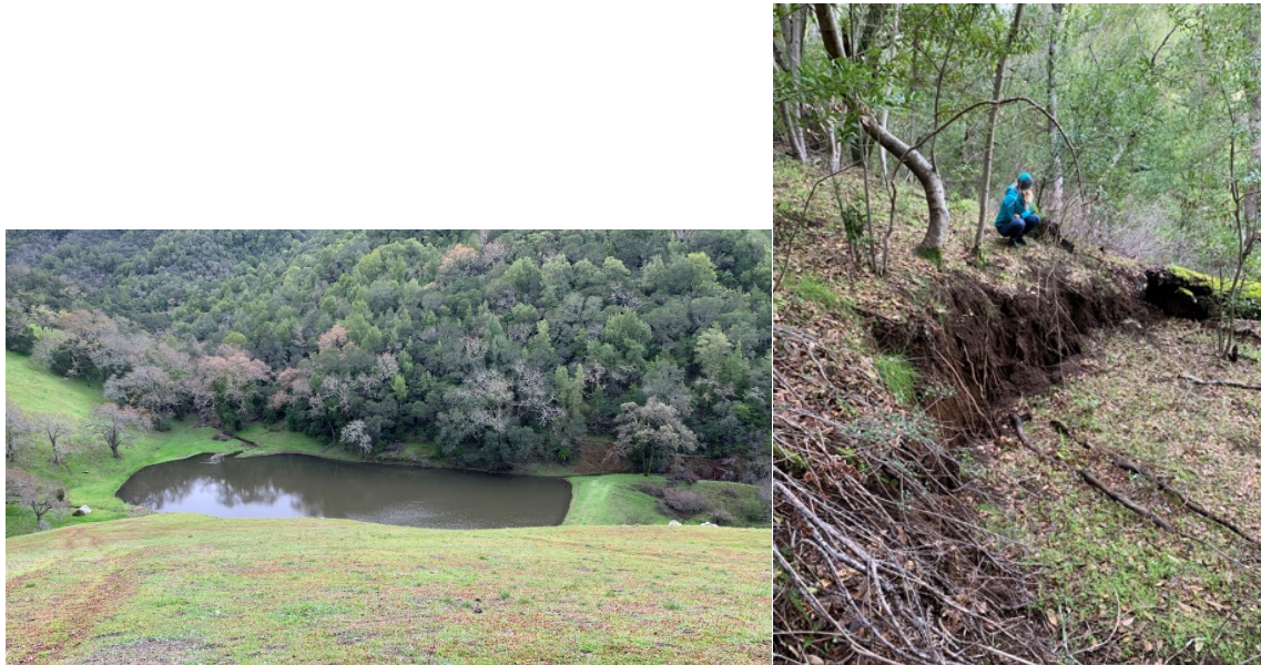
Figure 1. Pond RC-01 – Looking Down on pond from Assess Road, Landslide Head Scarp Observed Jan 2022 after Heavy December Rainfall
